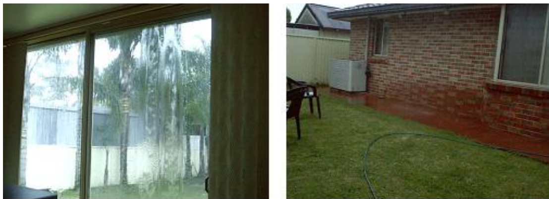
Figure 6. Curtain of water from overflow holes and splash line on wall.
